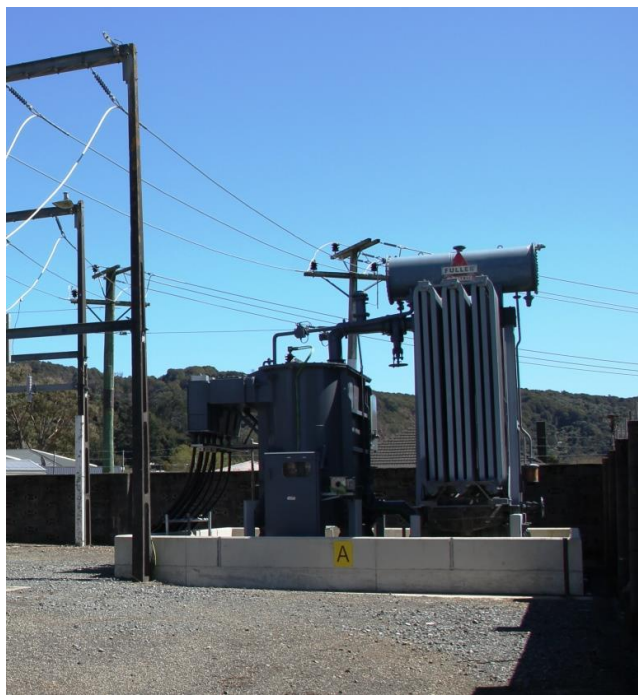
Zone substation power transformer
