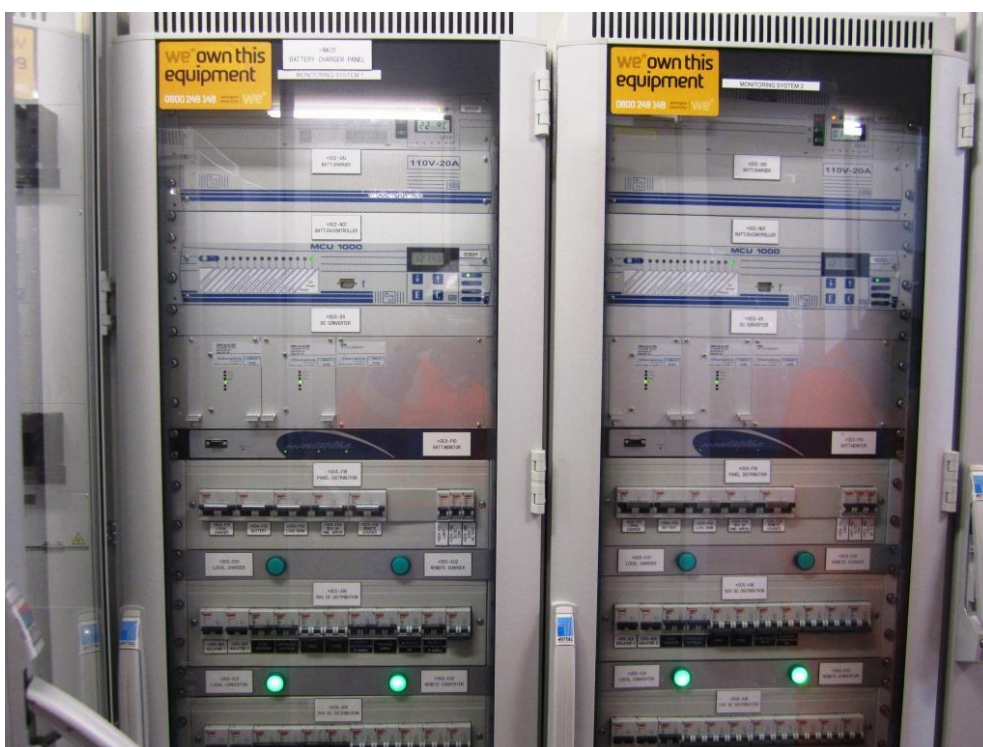
Substation DC panels
