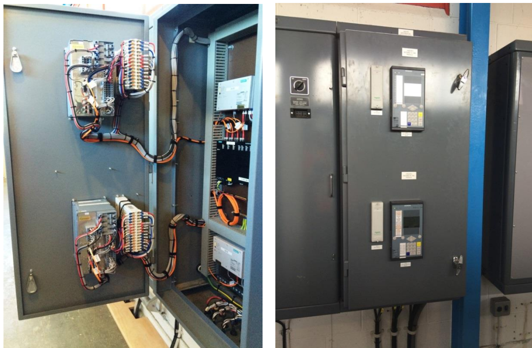
New protection relays
