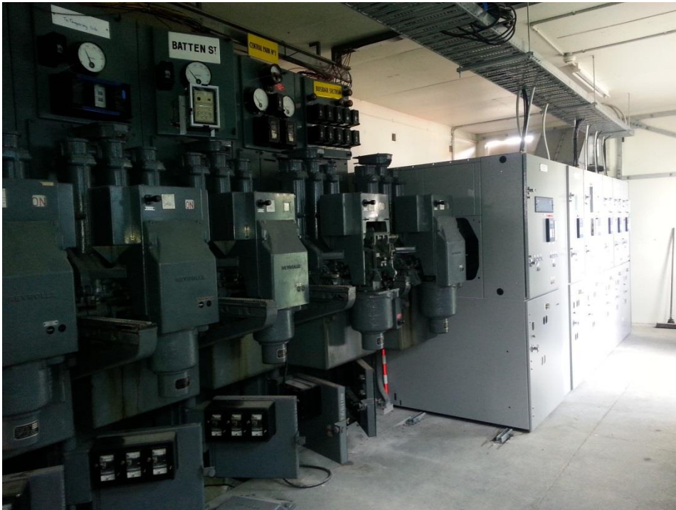
Replacement in progress of Reyrolle Type C with RPS LMVP switchgear at a zone substation
