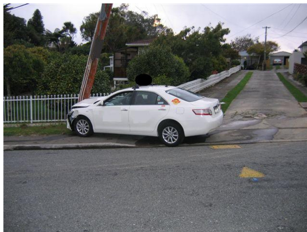
Network pole damaged following a car vs. pole incident
