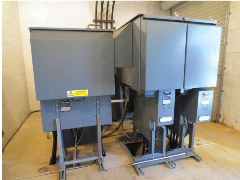
New indoor switchgear replacing SO-HI at an indoor substation
