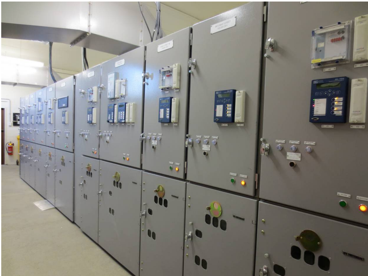
Palm Grove 11kV switchboard following replacement
