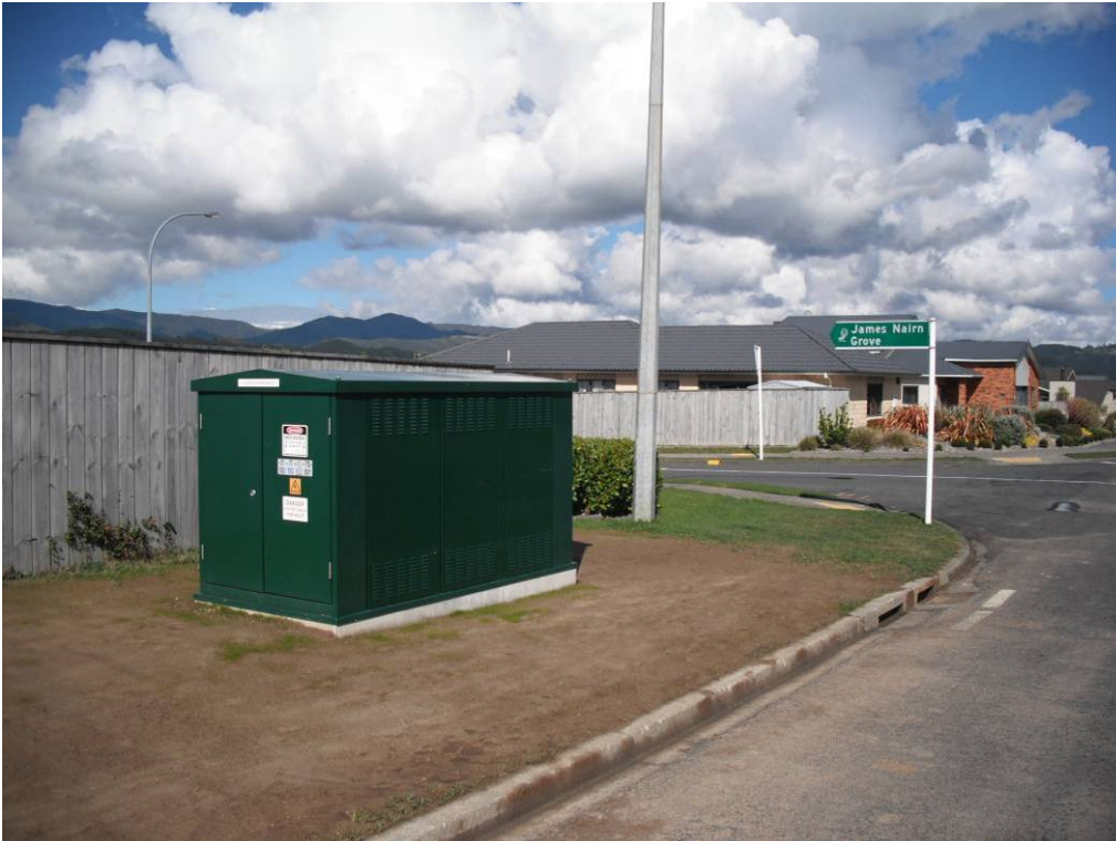
A new canopy type substation installed in a subdivision
