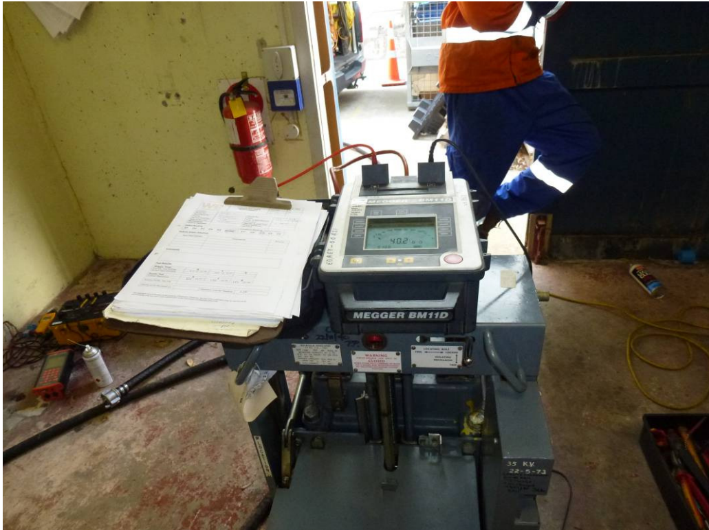
Circuit Breaker Testing in Progress
