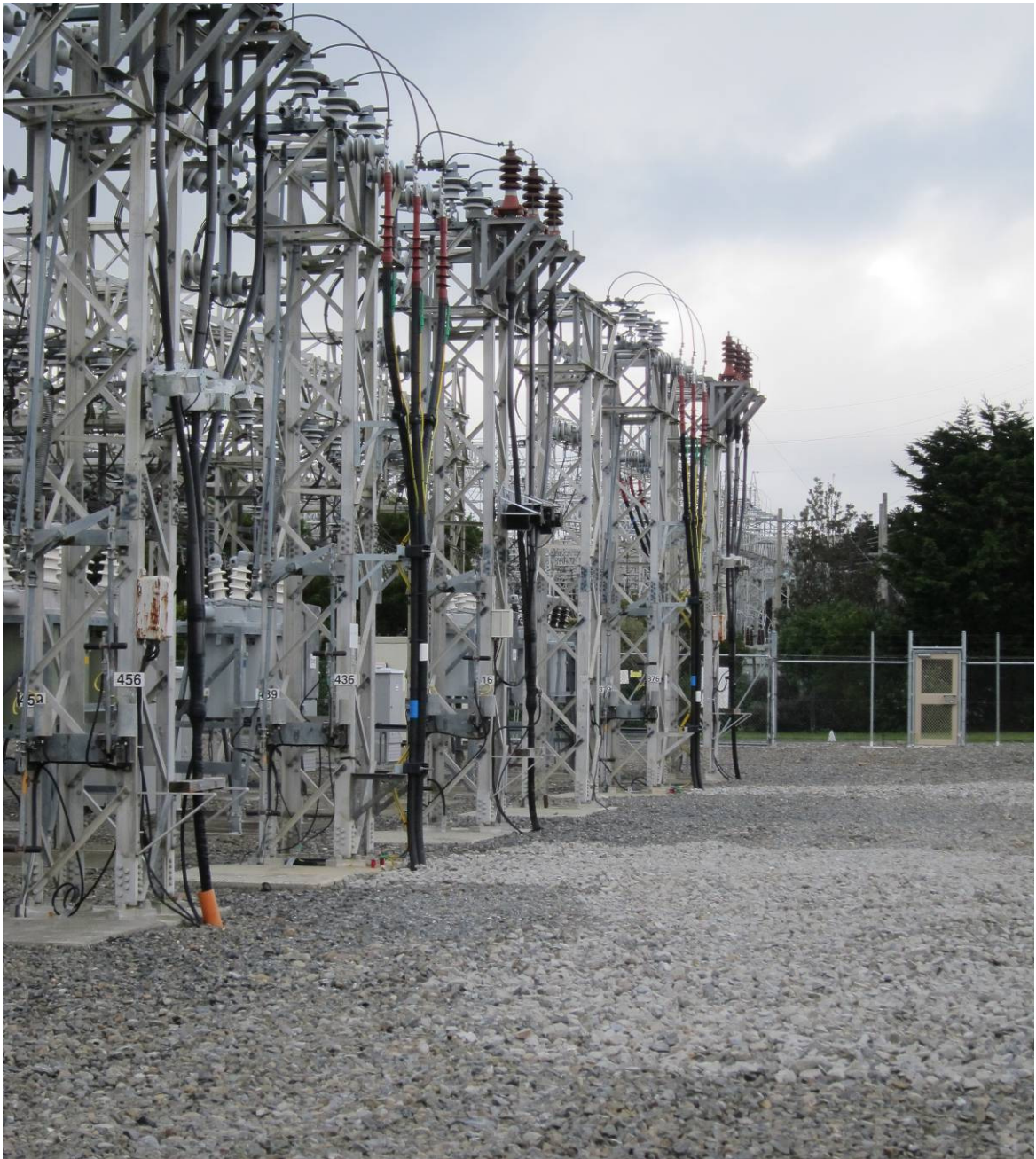
Subtransmission circuits leaving the Wilton GXP
