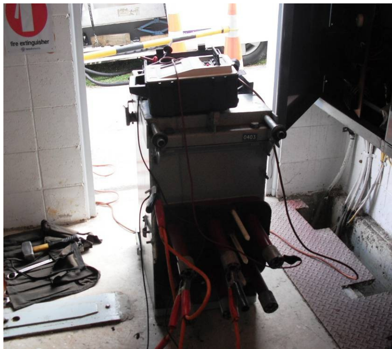
Testing of an 11kV circuit breaker carriage
