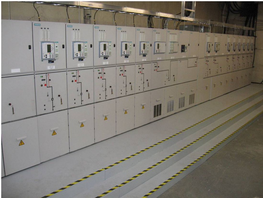
11kV Gas Insulated Switchgear at The Terrace Zone Substation
