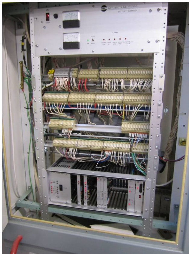
Plessey Dataterm RTU at Palm Grove zone substation
