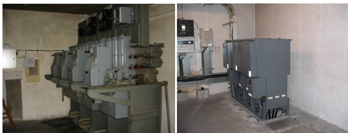
(L) Before and (R) After - Type C replacement at a Wellington Distribution Substation
