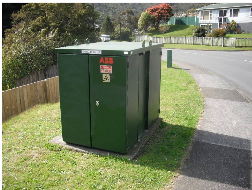
Typical Wellington Distribution Substation (Compact Berm type)
