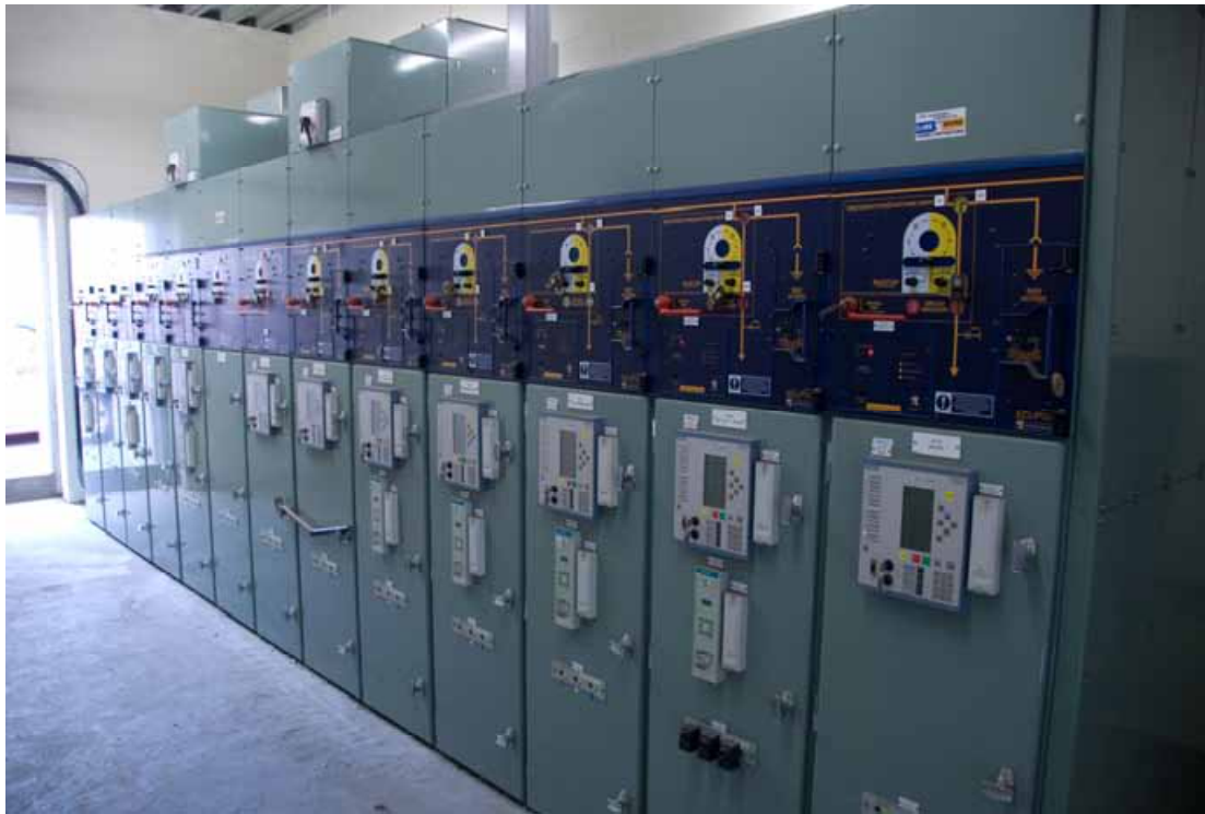
Switchgear in Thorndon Substation
