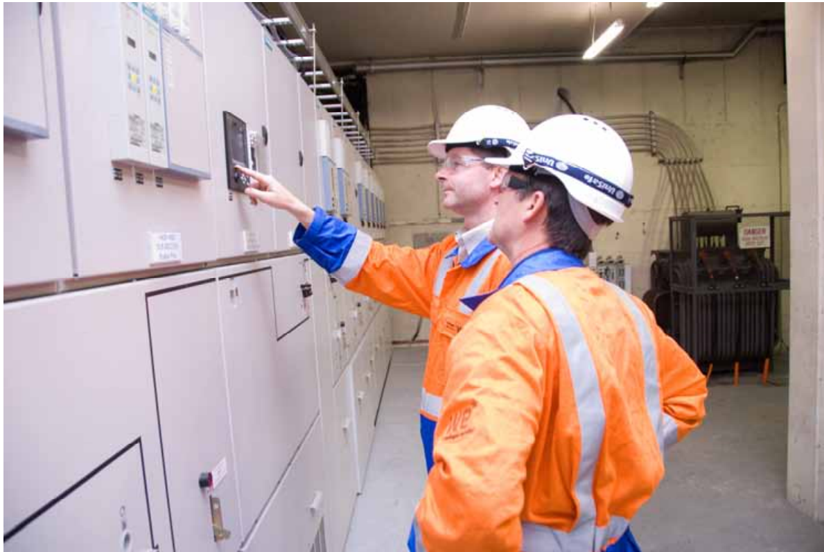
Switchboard in The Terrace Substation
