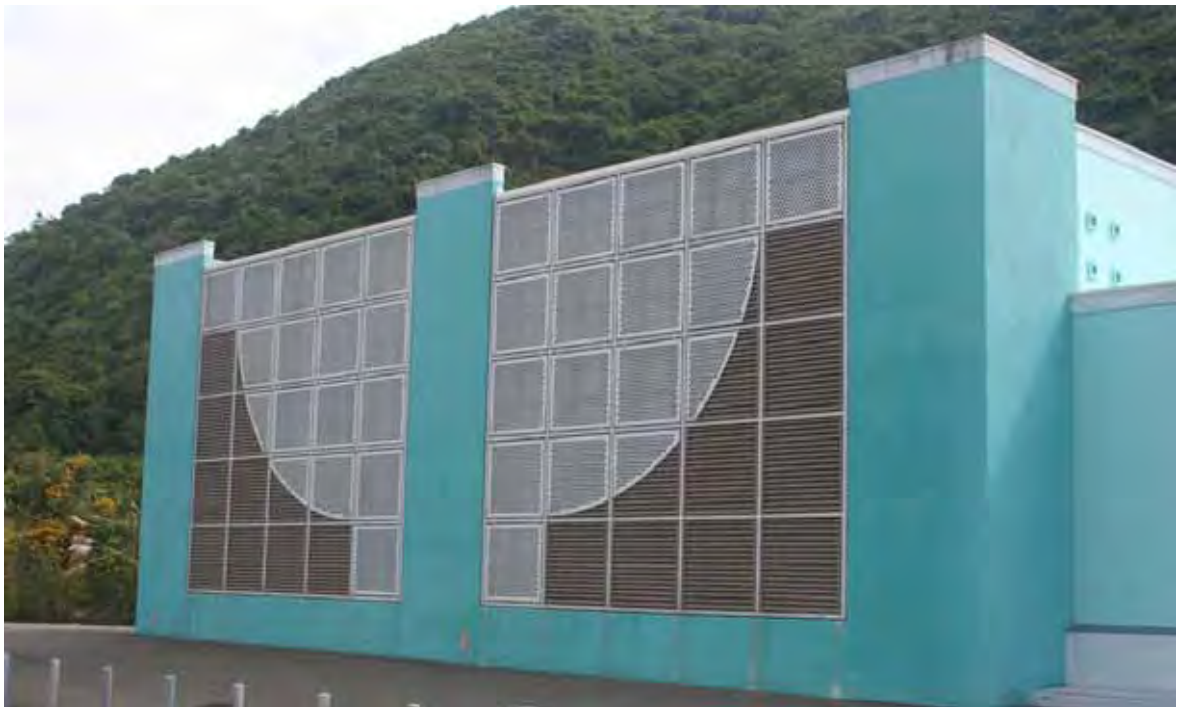
Ngauranga Zone Substation
