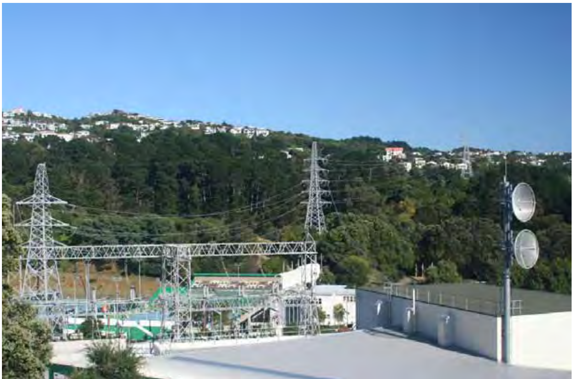
Transpower GXP Substation Supplying Wellington Electricity
