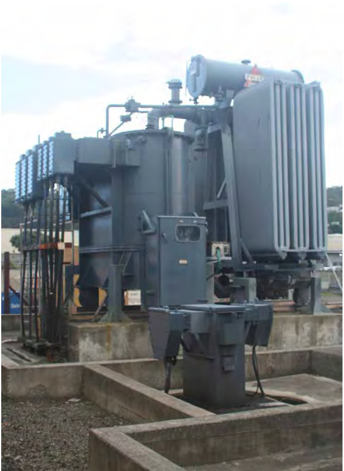
Petone Substation Transformer
