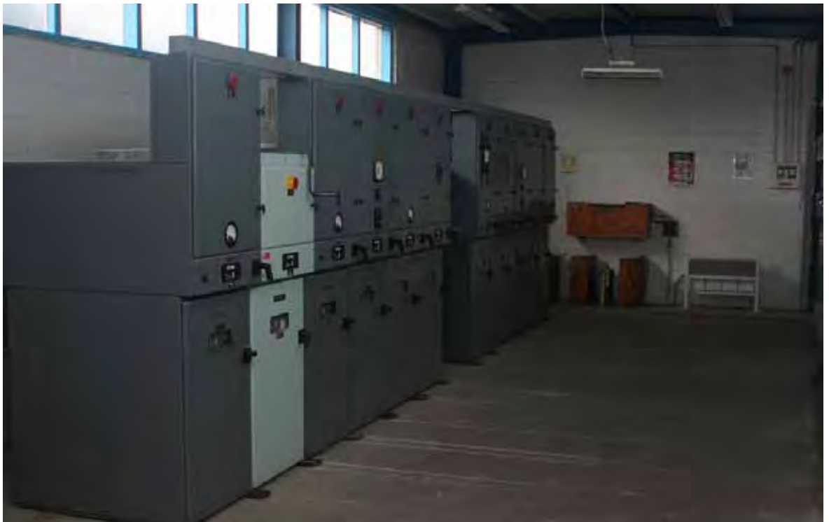
Petone Zone Substation
